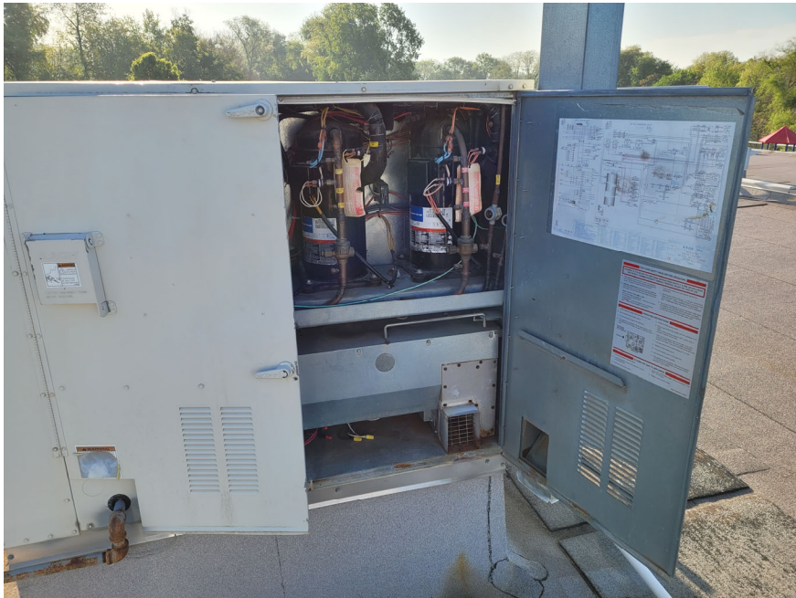
Rooftop unitary A/C
